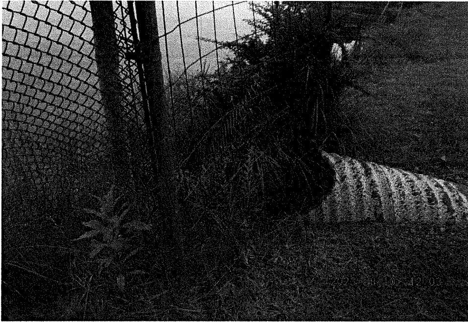
Photo 7 Dam ID# 163-0188 Treasure Lake Dam 08/10/2023 Auxiliary Spillway Inlet View: Right side of dam
