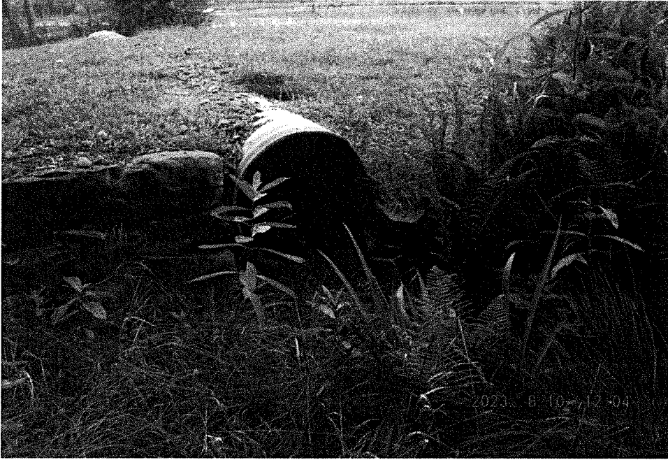
Photo 9 Dam ID# 163-0188 Treasure Lake Dam 08/10/2023 Auxiliary Spillway Outlet View: Right side of dam looking upstream
