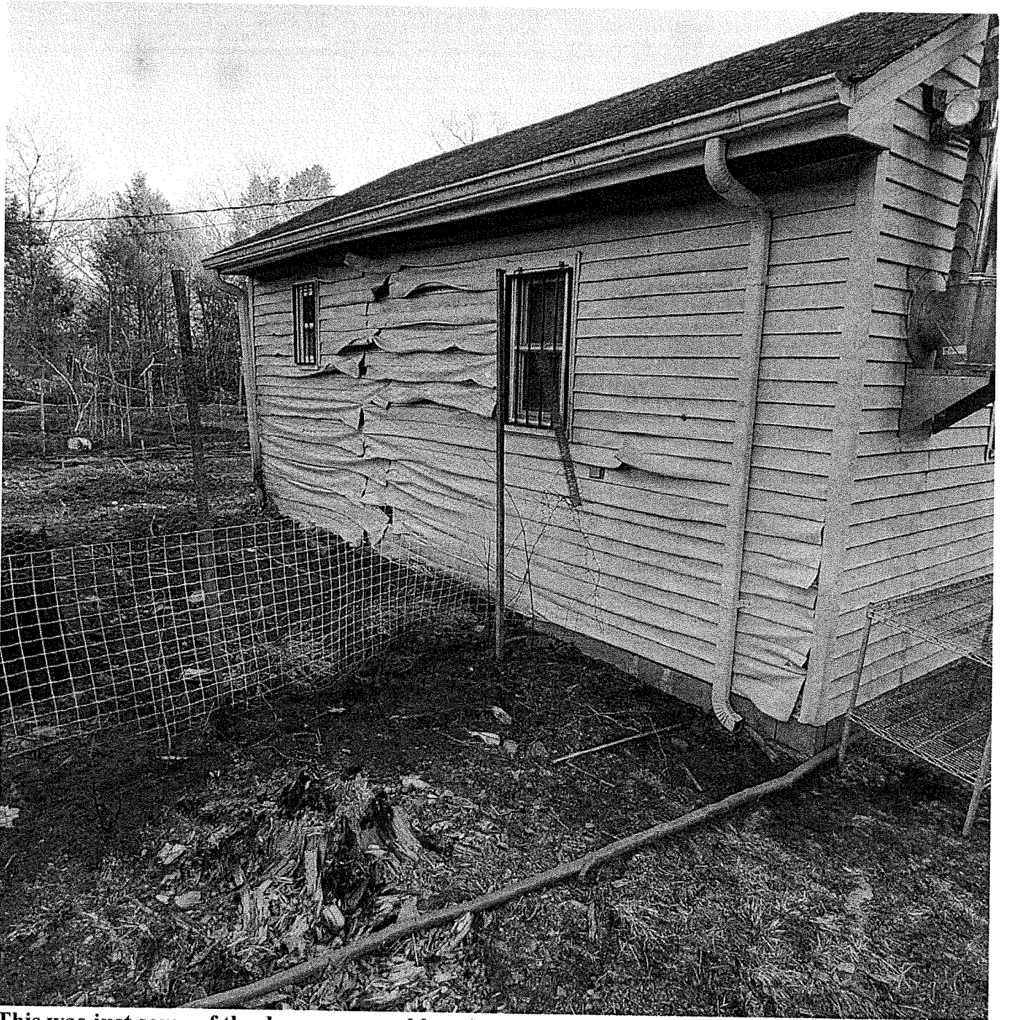
This was just some of the damage caused by a brush fire in Westbrookville a couple years ago, and local fire departments are bracing for numerous callouts, should residents not heed the current Statewide burn ban.
