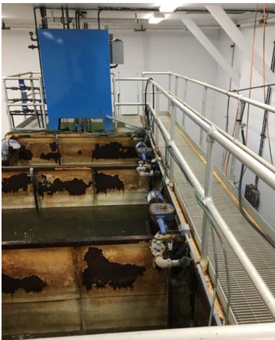
Sand Filter Interior
