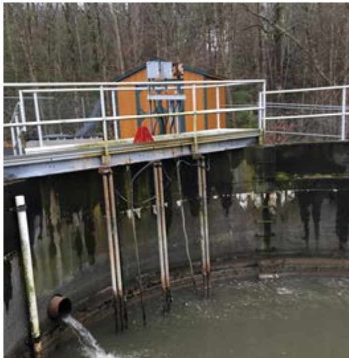
Influent Holding Tank
