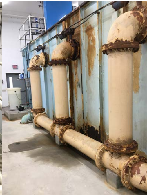
Sand Filter Exterior
