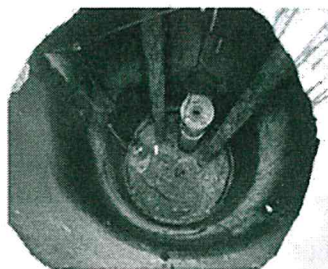
2 ½ feet of FOG in a wet well
